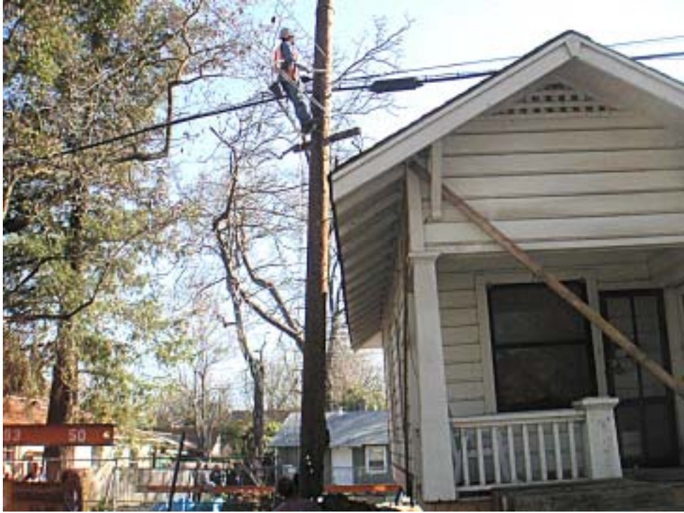
# 7. Getting the house onto the 516 D lot was delicate because the space between the electric pole on the left and the tree and house on the right only provided a few inches of clearance. Here we see the house clearing the pole on the left.
